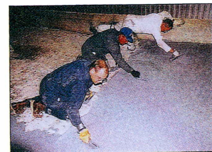
Proper Application: Tom Behunin (center) supervises hand-trowelling of ICO's epoxy coating applied at ConAgra's beef facility in Greeley, Colo. Preparation for this 2,200-square-foot job started at 7:00 a.m. The floor was back in use by 10:00 p.m. the same day.
