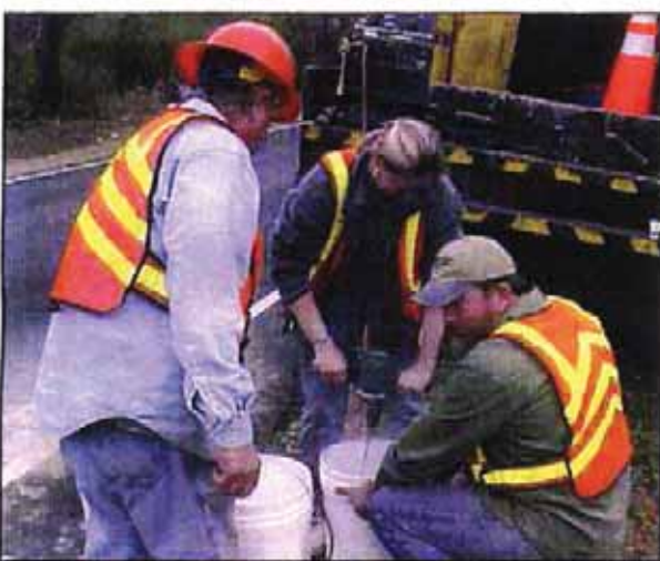
Prior to application, workers from the North Carolina Department of Transportation (NCDOT) mix patch material in the field.
